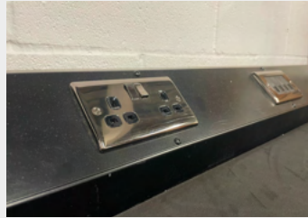
Worktop power and data channelling
